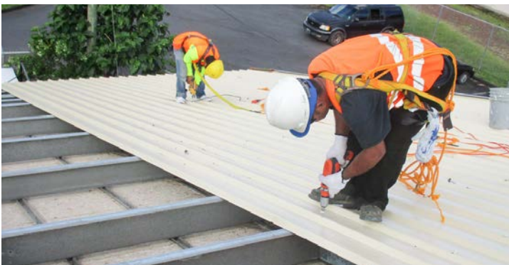
Workers from local contractor Global Tech Limited install new roofing on the cafeteria of Tafuna Elementary School
