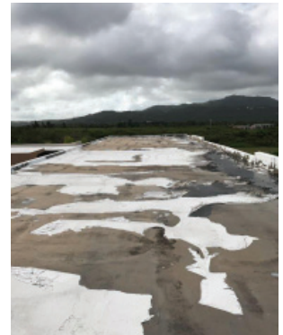
Roofing failure due to membrane delamination.
