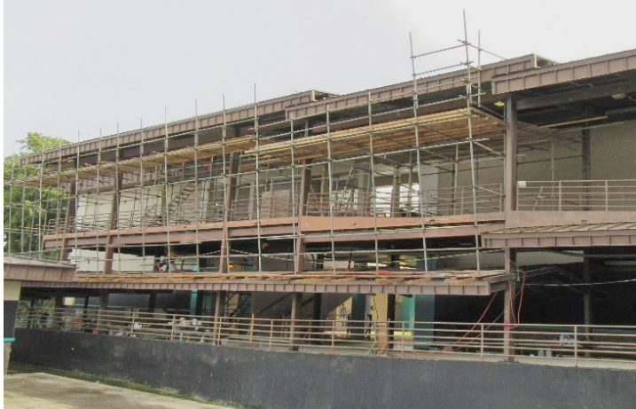
Structural repairs and new roofing to walkways in progress at Southern High School by local contract Bascon Corporation
