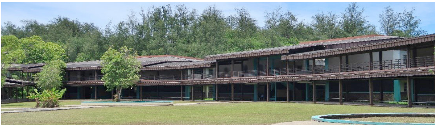
Completed walkway steel structural repairs and new roofing at Southern High School
