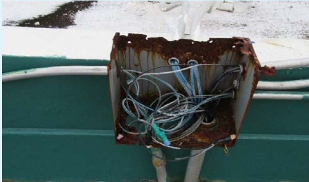
Rusted and deteriorated electrical pull box at Upi Elementary
