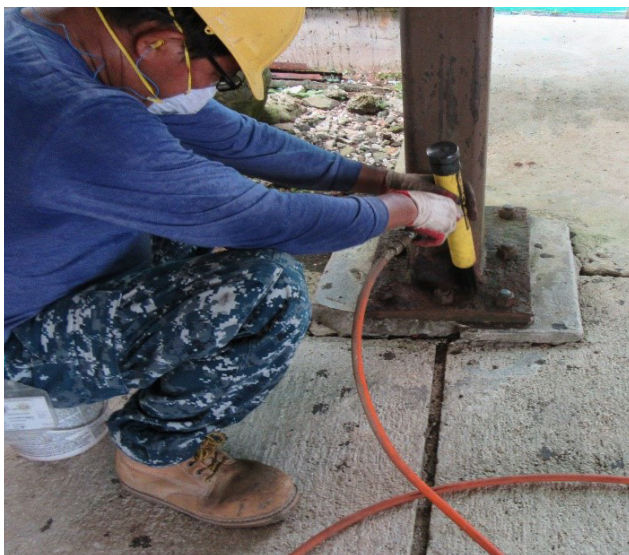
A worker from Bascon Corporation works on steel structural repairs on the covered walkways at Southern High School
